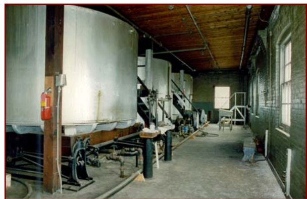
Building 58 & 59 4 th floor tank loft
