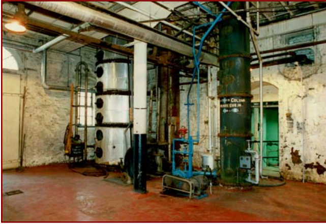
First Floor, Building 5, ca. 1986 by Larry Turner Badger distilling columns, southwest corner
