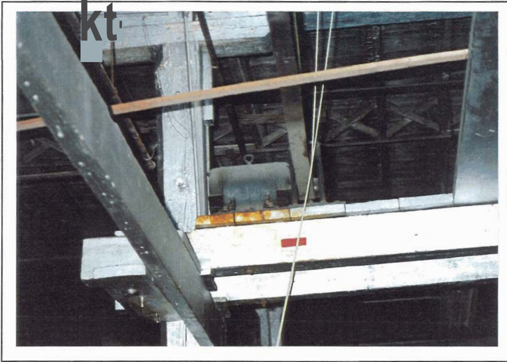
63-1-1 Air Compressor and Motor
